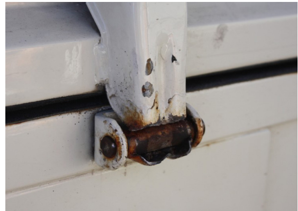
Figure 4. To retard its corrosion, this hinge is painted but the paint could not fully prohibit corrosion due to the cracks and holes within the coating. Moreover, part of the paint coating is peeled off
