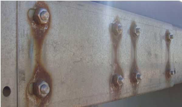
Figure 1. In this part of the food processing equipment, mild steel plate is combined with stainless steel bolts, giving rise to galvanic corrosion between the stainless and mild steel components
